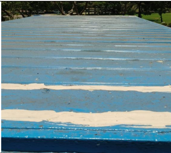
Fig 3. Container roof damage
