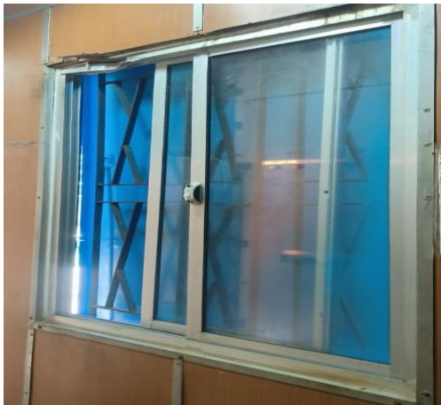
Fig1. Damage on window
