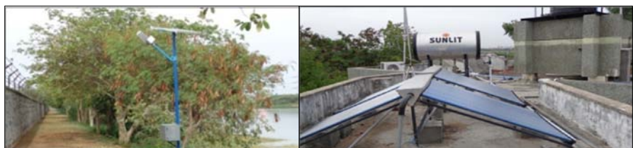
Newly installed solar lights near the compound wall
