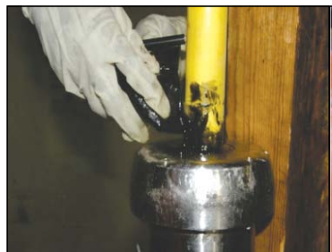
Electro-optic umbilical cable being re-terminated in TMS
