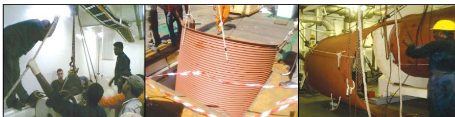
Upgradation of deep sea winch on board Sagar Nidhi
