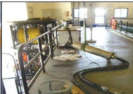
New slip ring being installed in TMS
